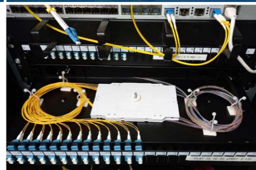
OLT Connection Splicing
