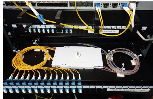
OLT Connection Splicing
