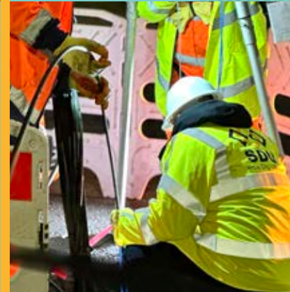
Fibre Optic Cabling
