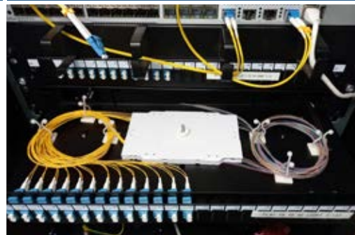
OLT Connection Splicing
